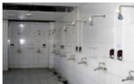
能耗监控系统 Energy Consumption Monitoring System
