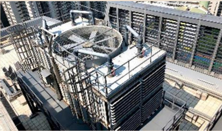
Modular cooling tower & condensing water pipework system
